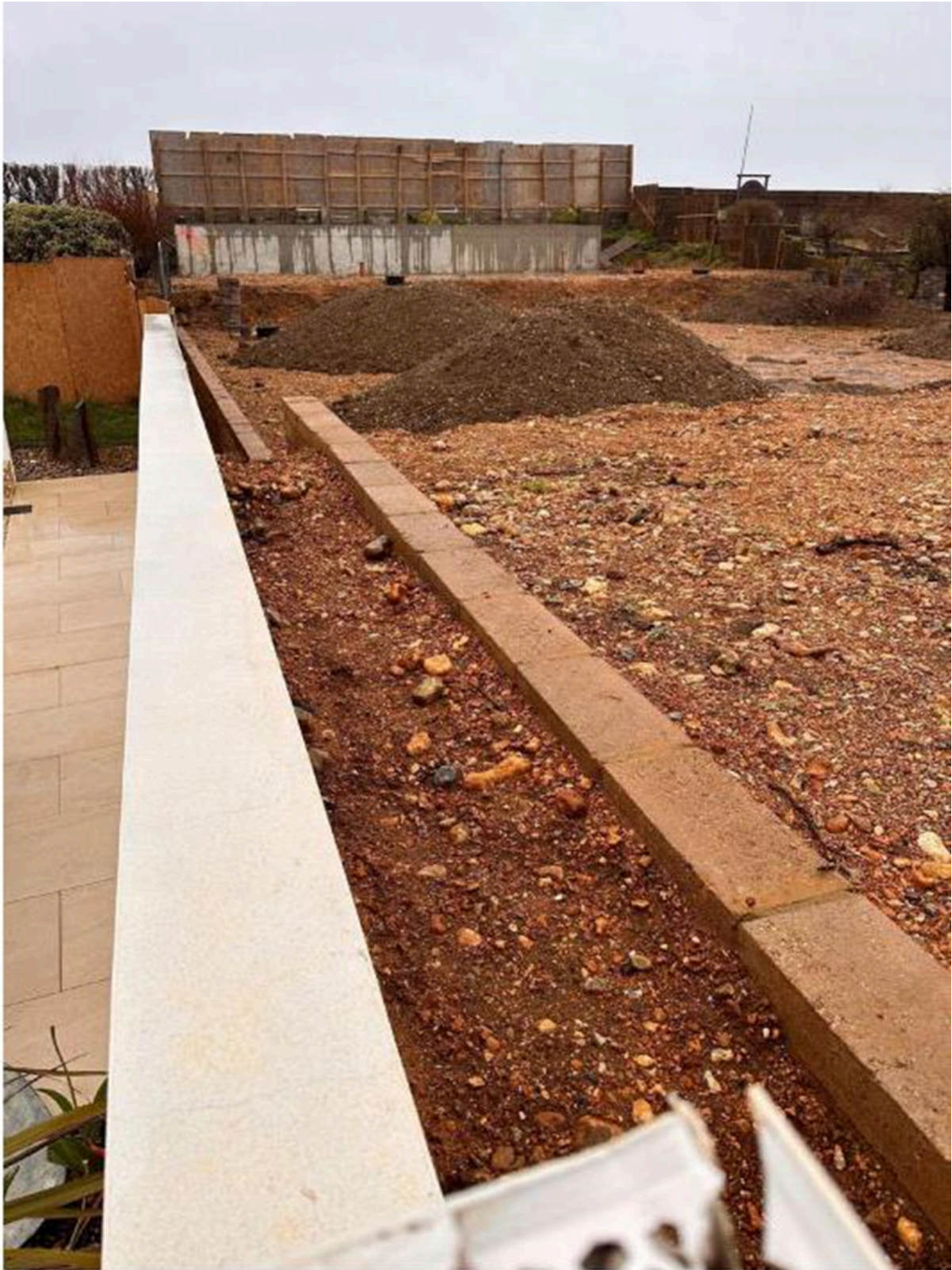
Images showing ground level of No. 44 to the left, and the raised ground level of No. 42 to the right.
